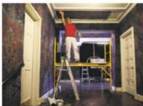
General contractor Tristan Harris hangs new wallpaper as part of the Hotel Durant's renovation.
